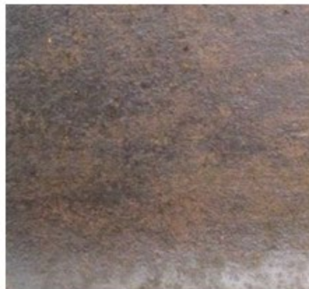
(f) 1948 rail (surface image of web)
