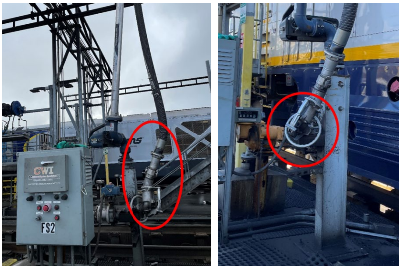
Figure 5. Example refueling receptacle diesel locomotives
