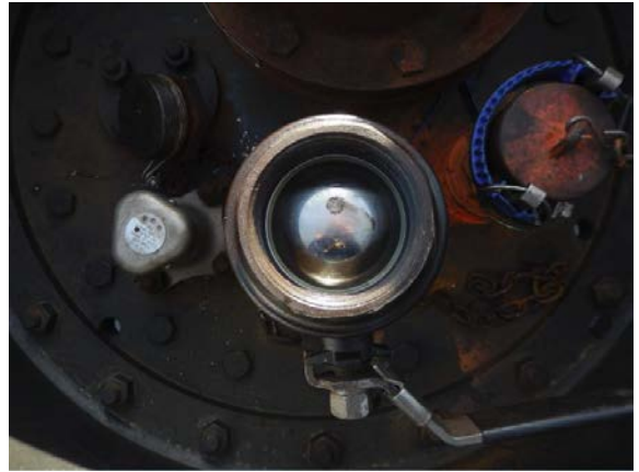
Impact mark on internal ball of valve evident of contact w/plug
