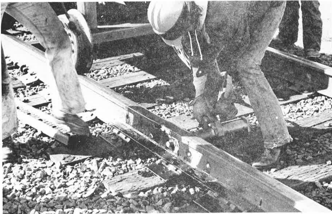
Figure 38.—Cold Expanding Joint Holes in the Field
