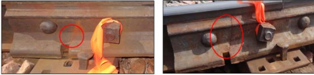
Figure 5. Quarter Crack and Quarter Break
