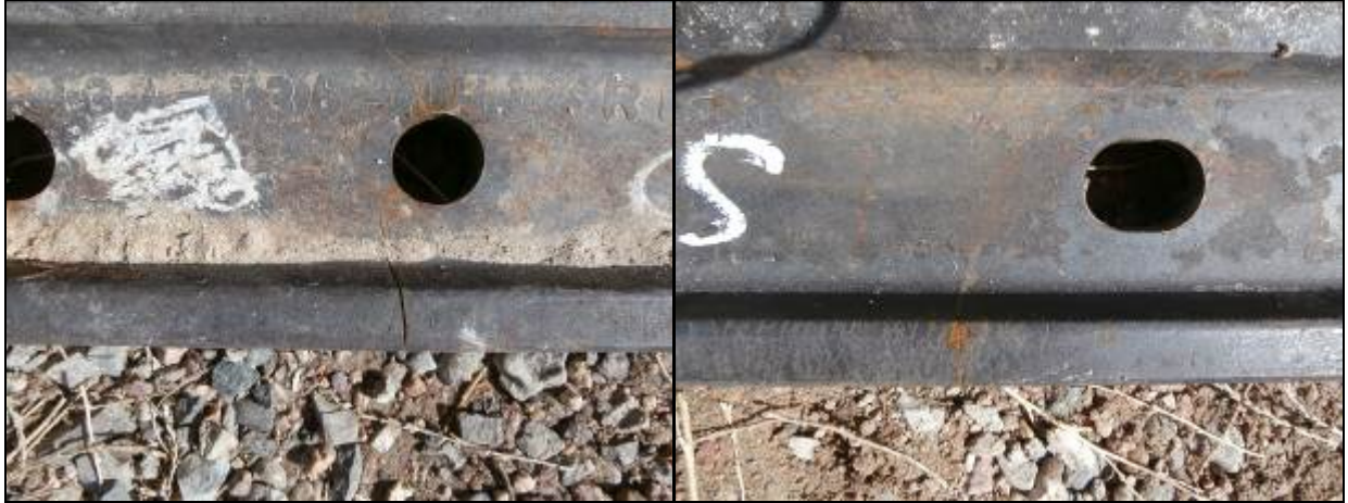
Figure 21. Fatigue Cracking in an Untreated (left) and a Post-Hardened (right) Joint Bar
