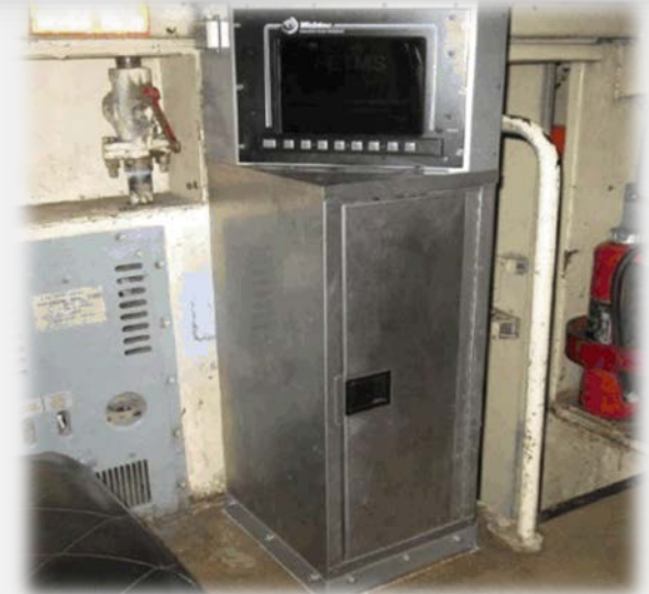
Example of retrofit components potentially blocking brake valve
