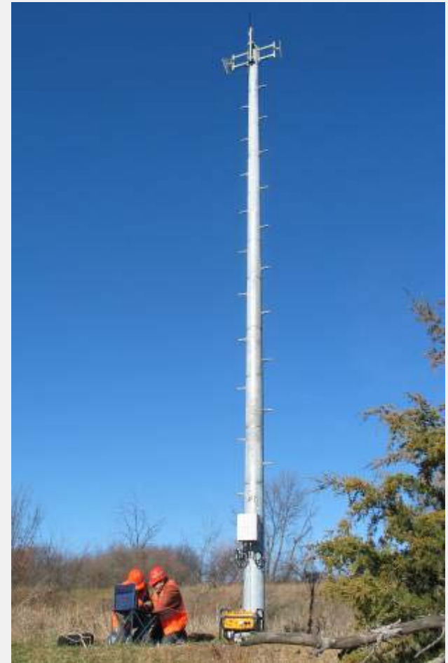
Example of a (small) communications tower
