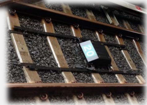
Examples of various methods for attaching transponders to track
